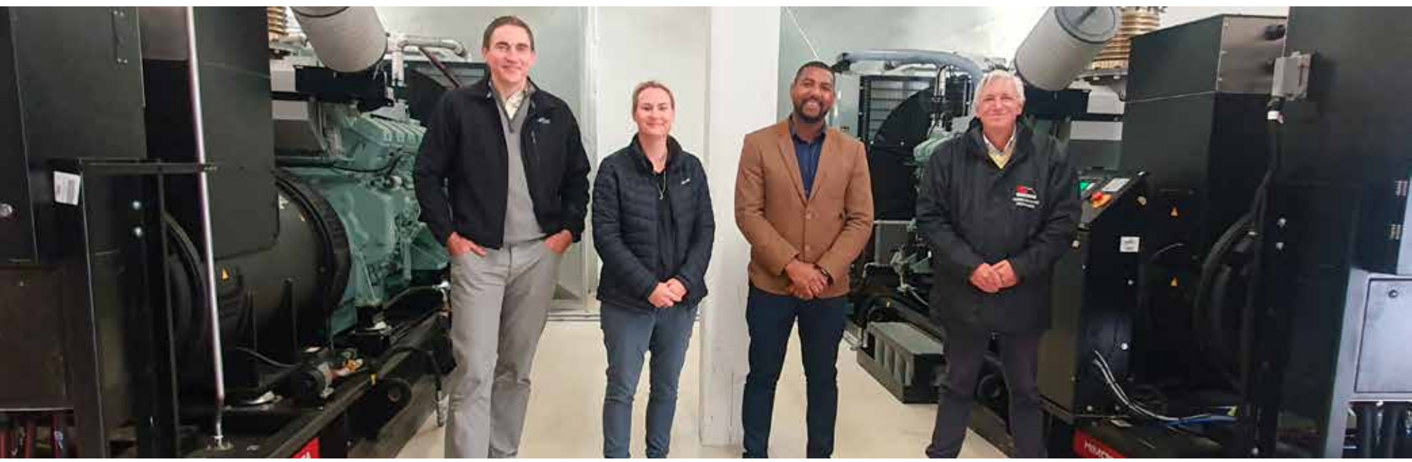
From left: Jannie Koegelenberg (Director of Civil Engineering Services), Councillor Jacquique Von Brandis (Portfolio Councillor: Civil Engineering Services: Capital Projects & BFI), Councillor Browen Johnson (Portfolio Councillor Civil Engineering Services: Operating Aspects), and Alderman Leon van Wyk.
