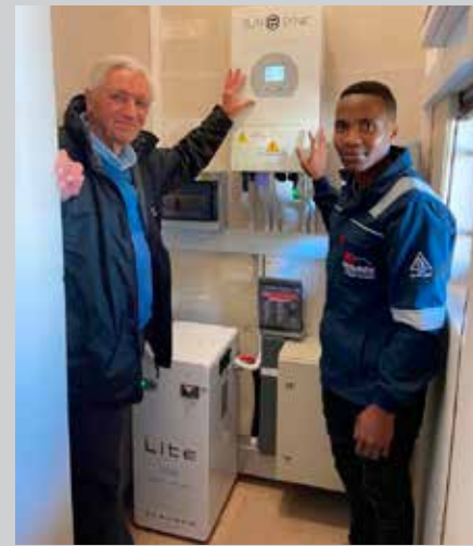
Blanco batteries: Mayor Leon van Wyk and Thabo Yiga, Project Manager of the Solar Systems at Electrotechnical Services at the batteries for the solar system installed at the Blanco Drive-through MVR.
