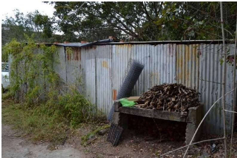
Picture 3. Existing dilapidated shed
