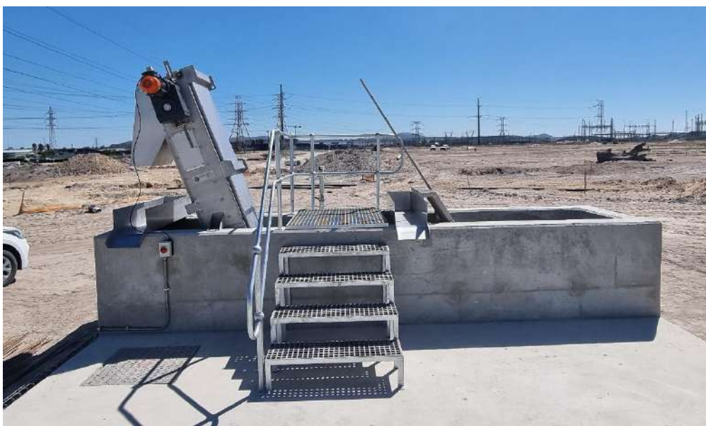
Figure 3: Concrete underground MBR Treatment Plant Inlet Works
