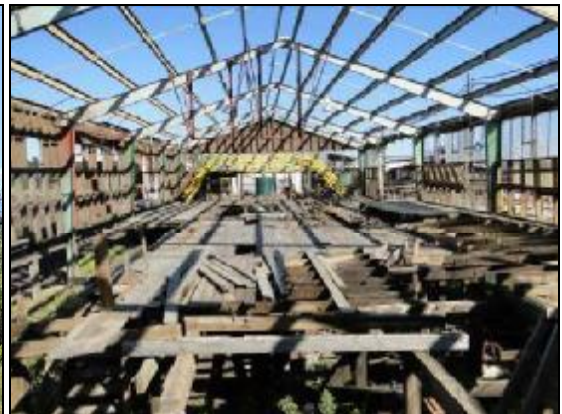
Image 7: Remaining interior of timber structure
