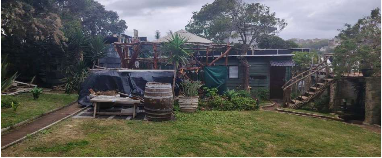
Photo 5 This photo shows the existing domestic worker room (on the right) and the unfinished toolshed (left side of photo). Note that all these buildings (including the timber deck and stairs seen on the right side of the photo) were demolished in the meantime and the material lying round on the erf, removed from the erf. See photo 6 below.
