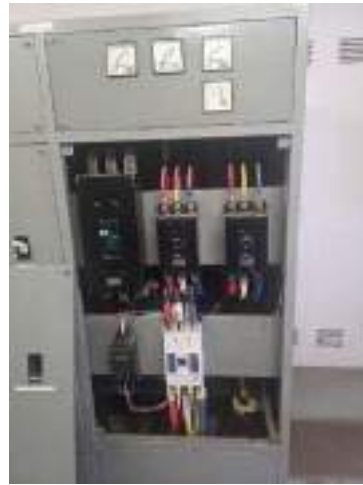
Fig 4 LV Panel to be upgraded
