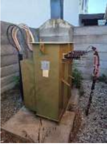
Fig 1 Transformer to be replaced
