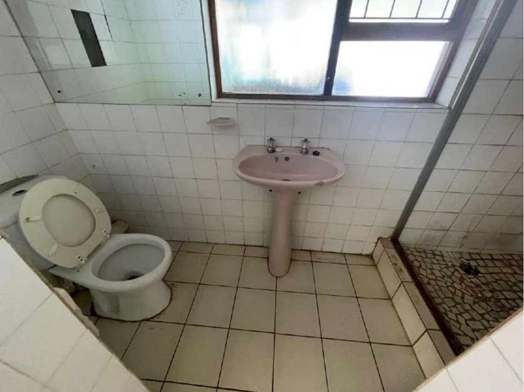
Damaged and moldy tiles, as well as plumbing not repairable and will need to be completely re-done .
