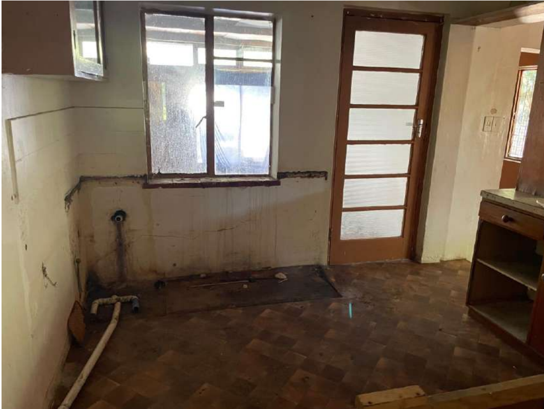
Plumbing and electrics are not repairable and will need to be completely re-done.
