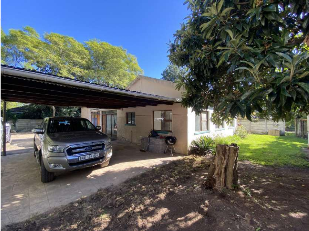
Front of house with shaded parking area –roof of covered parking is rusted and fascia’s rotted
