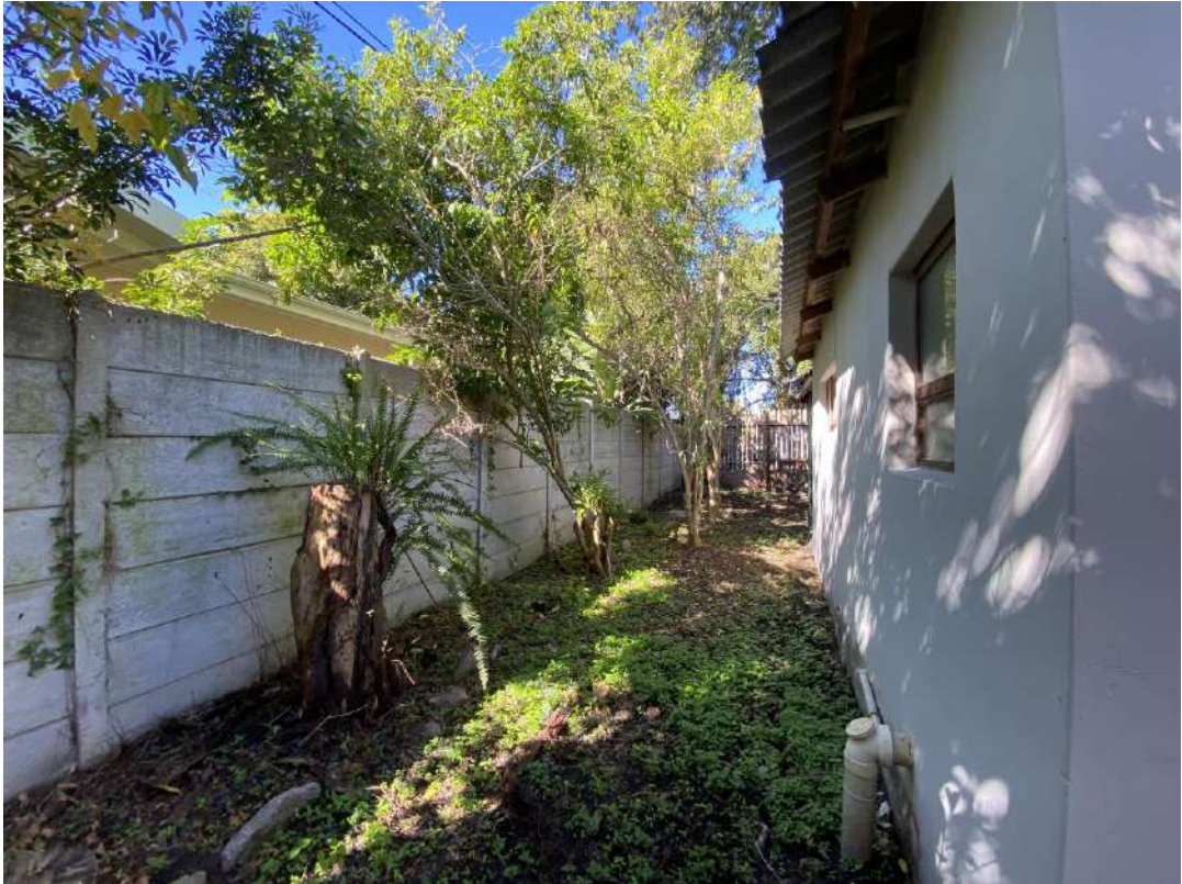
Back of out building next to house and dilapidated vibacrete boundary wall
