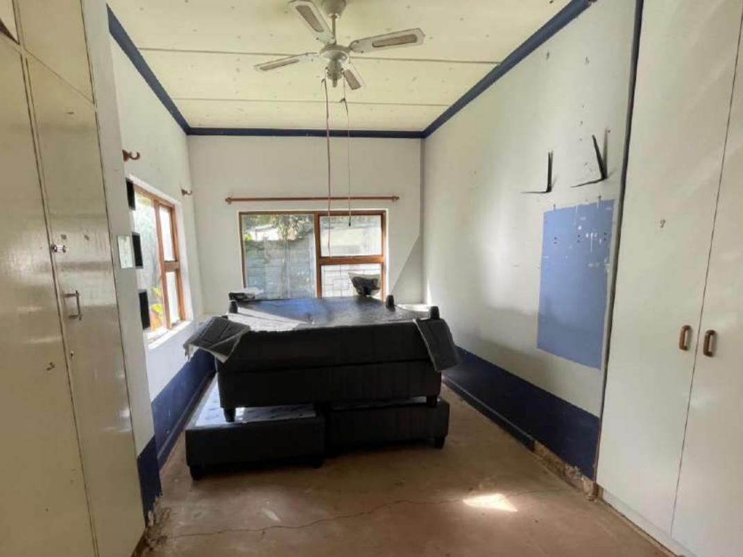
Skirtings and joinery damp and disintegrating.
