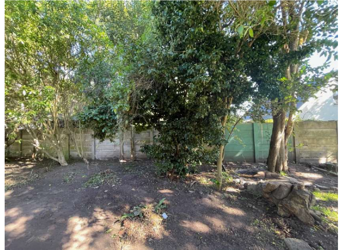
Trees on west side boundary with dilapidated vibacrete wall
