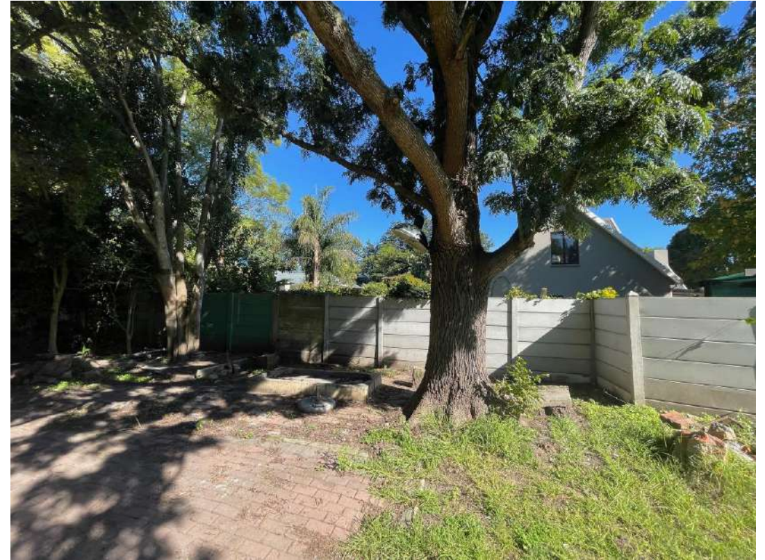
Trees on west side boundary with dilapidated vibcrete wall
