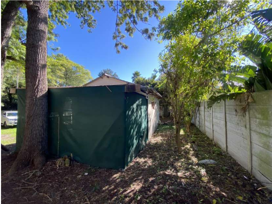
Poorly constructed temporary structure
