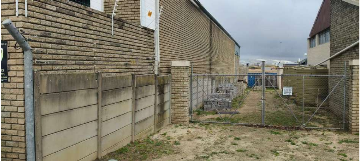
Photo 6 The photo shows a building in the industrial area that was erected on the boundary of the erf. Note that the 1.8m high boundary wall on the adjacent erf serves no purpose as the wall of the building actually performs the role of a boundary wall that exceeds the height of the permissible 2.1m wall by far – much more than 2.4m as requested in this application.
