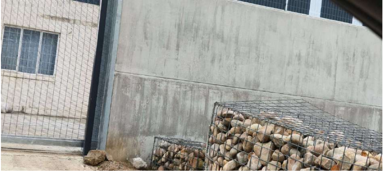
Photo 2 This photo is a zoomed-in version of photo 1 to show the joint between the two 1.2m wide concrete slabs of the wall more clearly.
