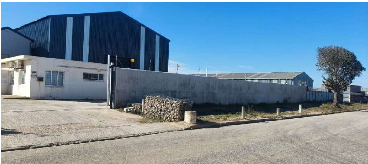
Photo 1 The photo shows the wall along Ring Road on the most eastern side of the erf. If zoomed in, the joint between the 2 concrete slabs on top of each other, is clearly visible. The building on the erf, is the latest addition for which an occupation certificate must still be issued. Also see Photo 2 below.
