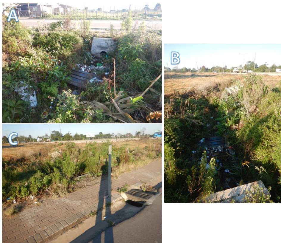
Figure 5: Photographs showing stormwater headwall discharging into Erf 7397 from Church Street (A); excavated stormwater canal running from Church Street along Erf 7397 towards Beach Road (B) and stormwater inlet on Church Street (C).
