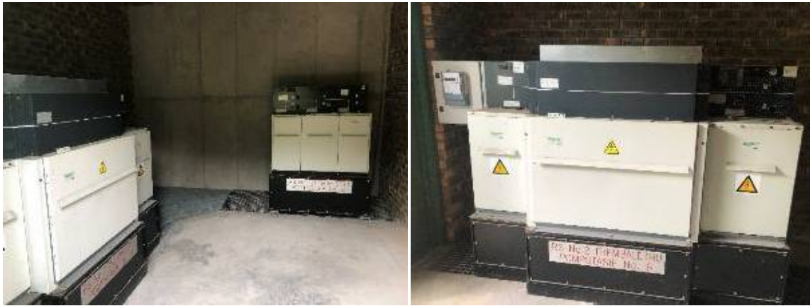
Figure 3-13: Existing Medium Voltage Metering Unit
