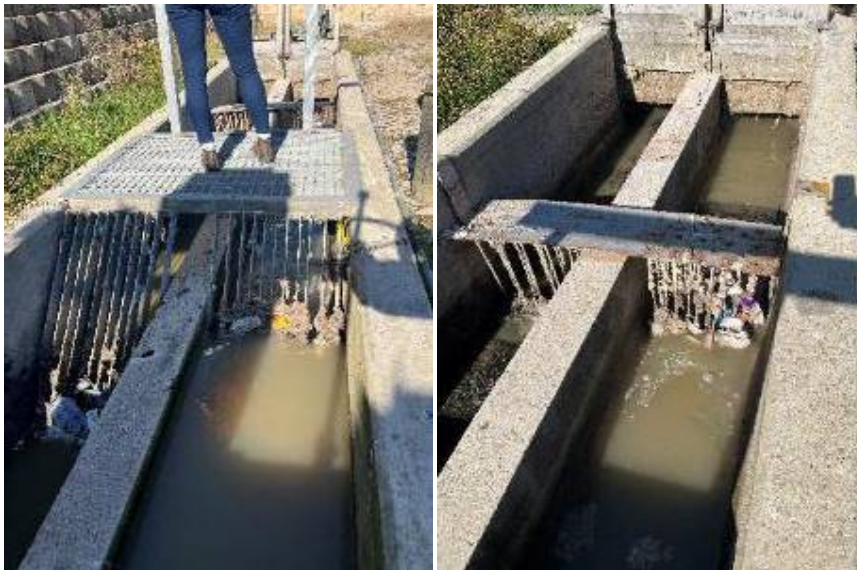
Figure 3-6: Existing hand rake screens
