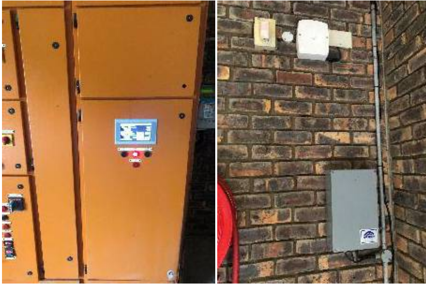
Figure 3-18: Existing Telemetry & Control Panel
