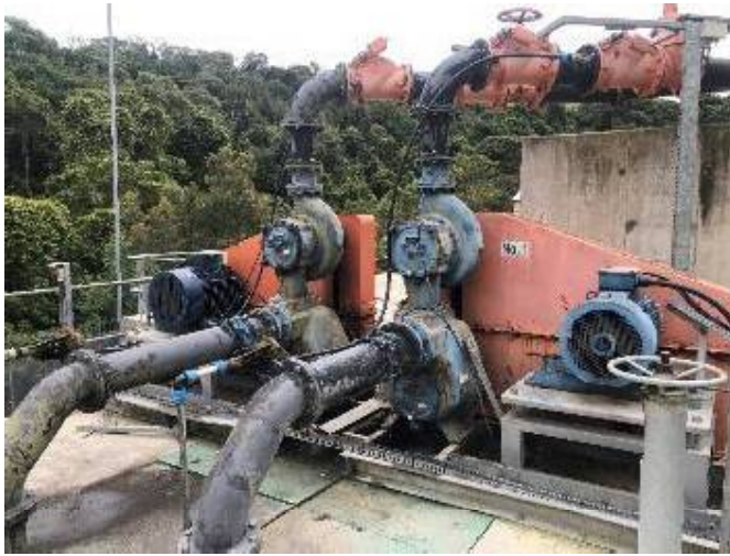
Figure 3-16: Existing LV Motors
