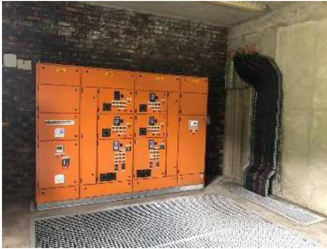
Figure 3-15: Existing LV Motor Control Centre
