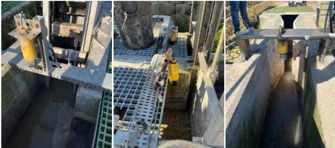
Figure 3-7: Existing ultrasonic flow measurement
