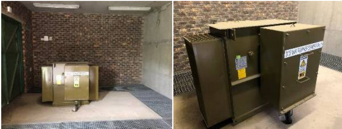
Figure 3-14: Existing Power Transformer No.1 (315kVA)
