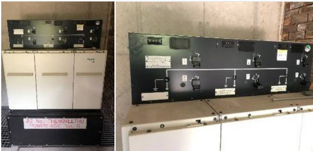
Figure 3-12: Existing Medium Voltage Ring Main Unit
