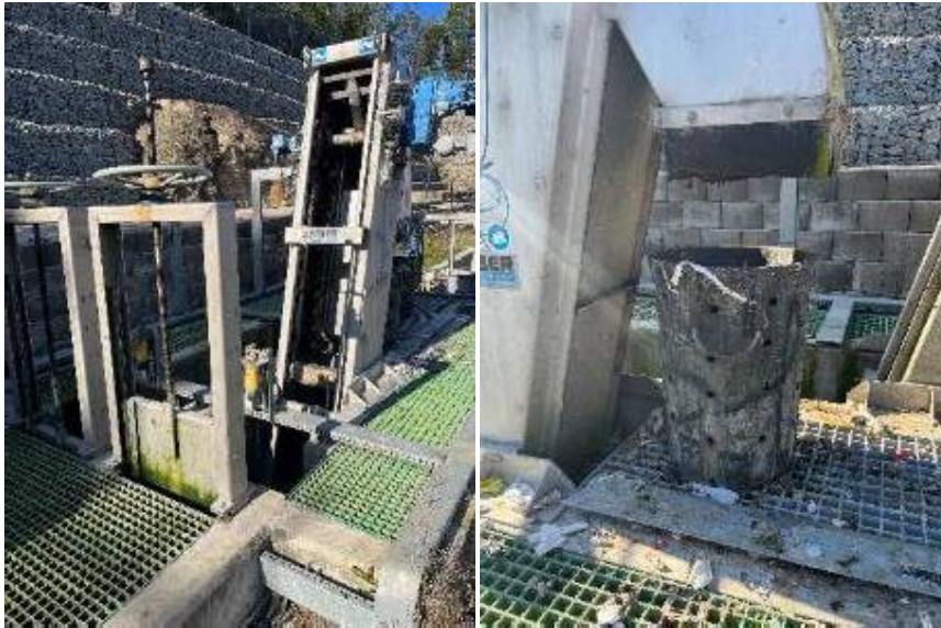
Figure 3-5: Existing mechanical screens
