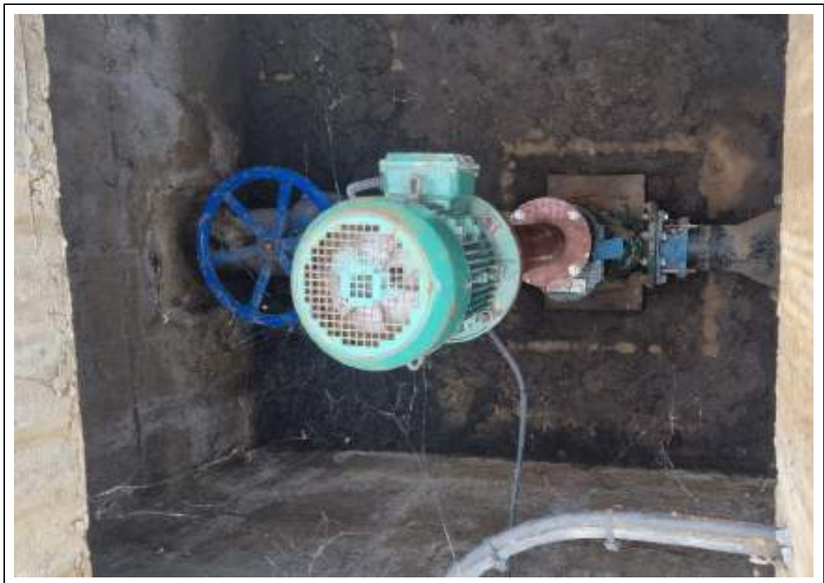
Figure 6 : Picture of the Inline Macerator Unit Installed in the Pipe Chamber
