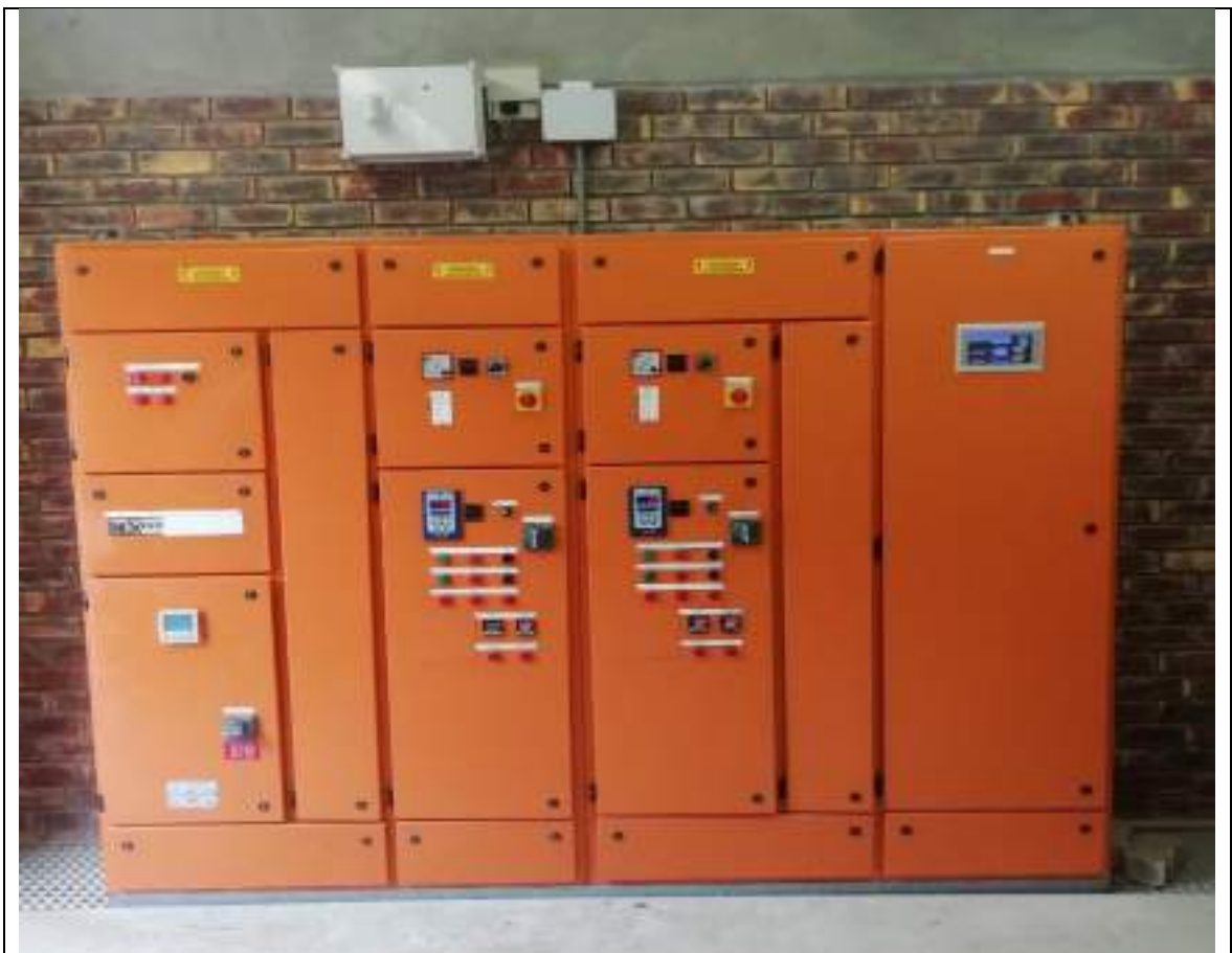
Figure 10 : Picture of the Existing Pump Station MCC unit
