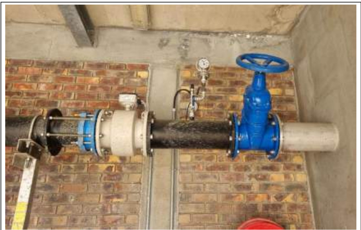
Figure 8 : Picture of the Existing Siemens Flow Meter Installed in the Pump Room
