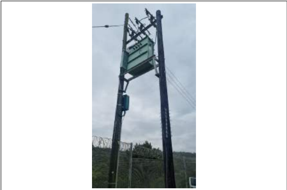
Figure 11 : Existing Pole-Mounted Transformer
