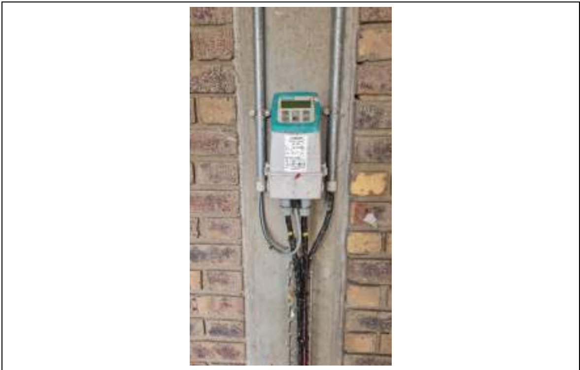
Figure 9 : Picture of the Flow Meter Display on the Wall in the Pump Room below the Flow Meter
