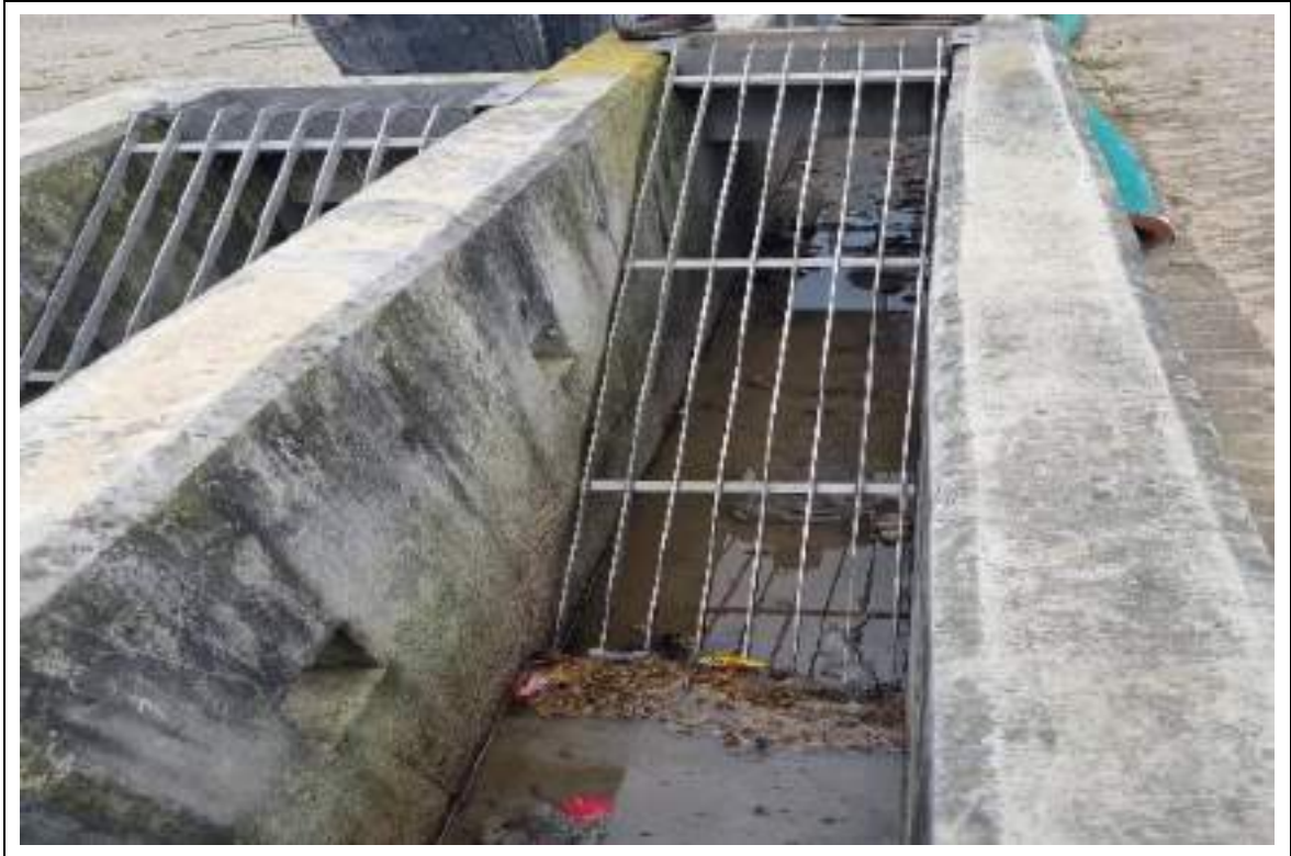
Figure 5 : Picture of the Manual Hand-Raked Screens Installed in Screenings Channels
