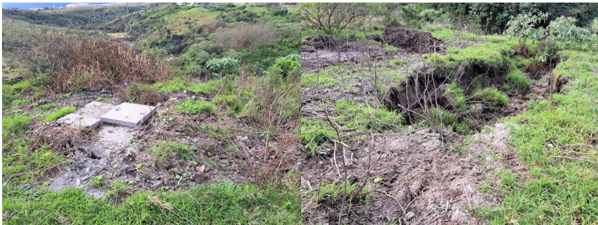
Figure 4-9: Example of a blocked sewer manhole (left) that caused erosion down the embankment to the river (right).
