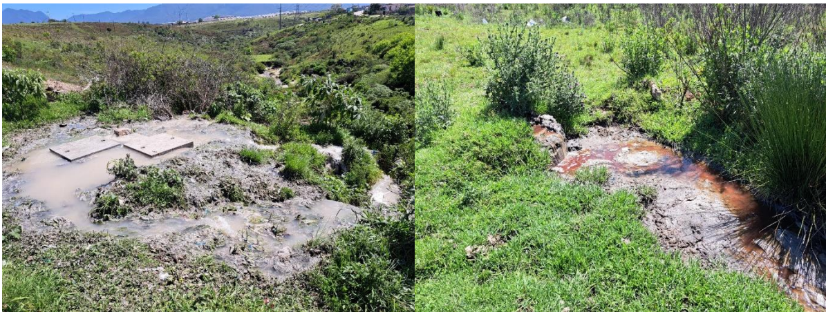
Figure 9-3: Two examples of leaking manholes along a 500 m stretch of the Schaapkop River
