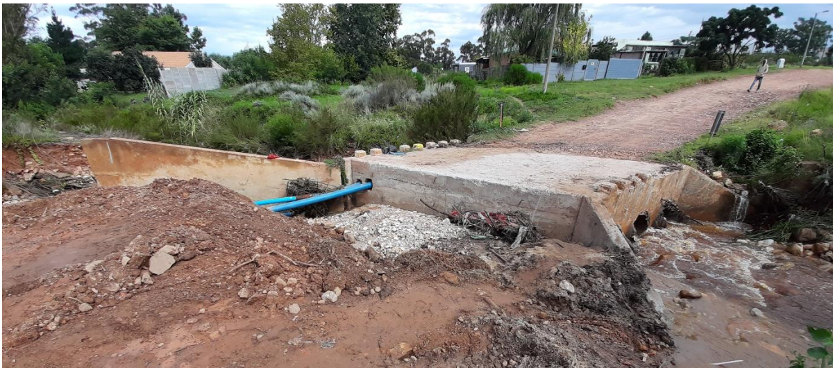
Figure 5-3: Example of a combination of multiple failure types (not in study area, for illustrative purposes)
