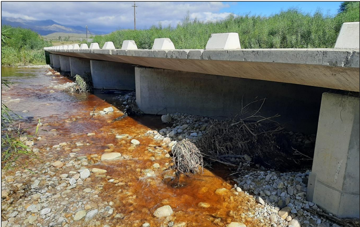
Figure 5-5: Road bridge design and/or function being impacted by debris (not in study area).
