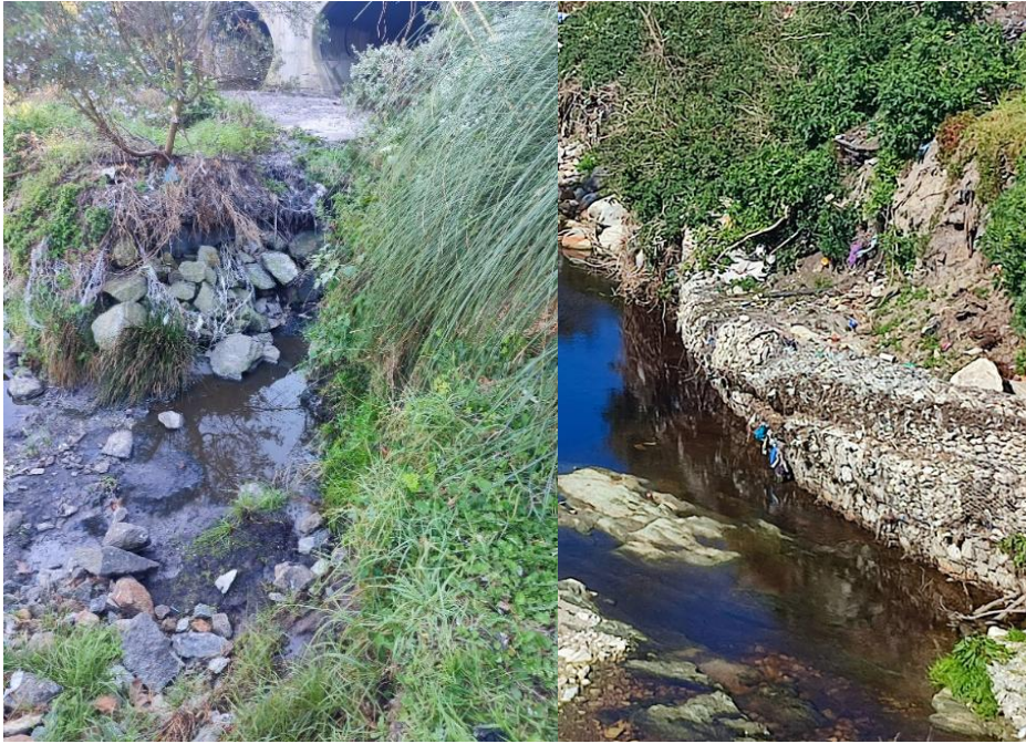
Figure 5-2: Structural failure but still functioning.
