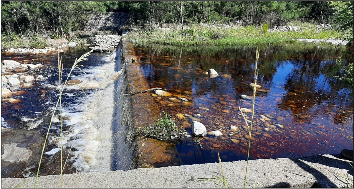
Figure 5-4: Water retaining structure (storage) compromised due to infilling by debris (not in study area).
