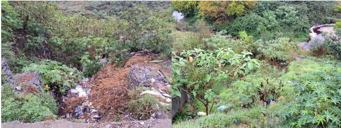
Figure 4-8: Photographs illustrating erosion of embankment down to Schaapkop River at stormwater outlets.
